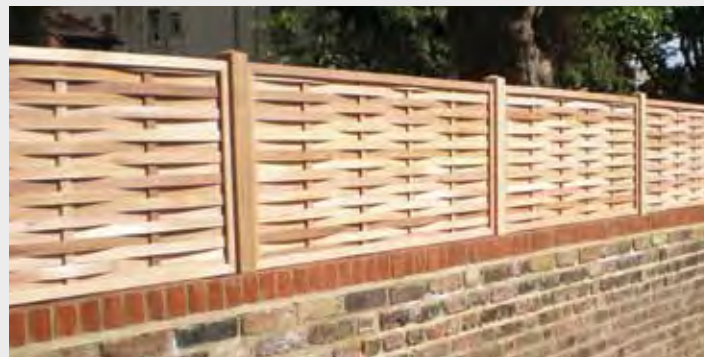
▶ RIGHT Cedar weave fence panels fitted on top of an existing brick wall.
